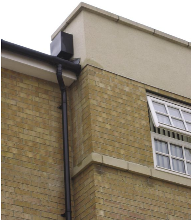
Poor rainwater detailing, leading to leaks, dampness and staining.
