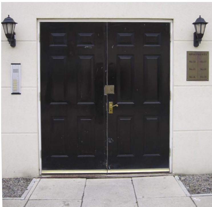
Inadequate door specification and poor workmanship led to maintenance problems after only two to three years.
