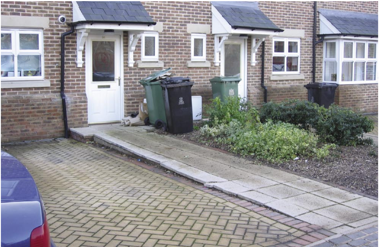
Inadequate detailing and poor workmanship to external works, and lack of bin stores.
