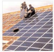
Photovoltaic roof panels
